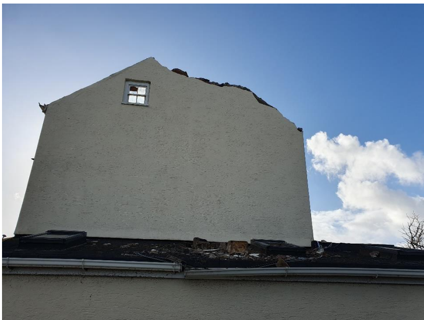
Figure 47: View of northern and eastern faces of Greycliff Cottages, showing partial loss of the gable wall.
