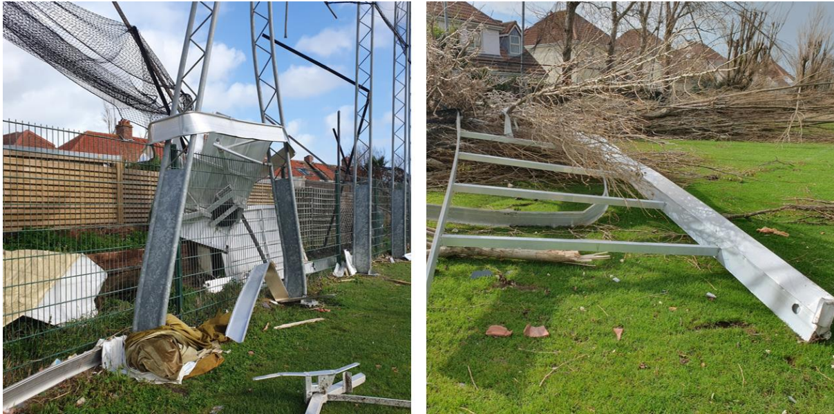
Figure 16: Metal structures torn and twisted at the southern side of Florence Boot Playing Fields.
