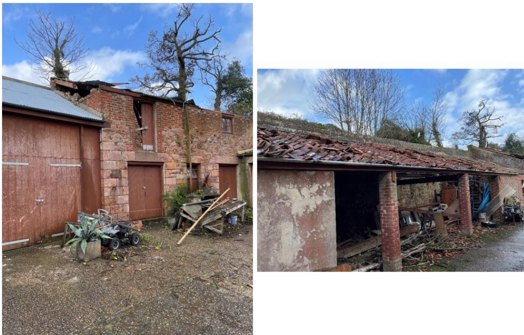
Figure 35: North barn (Figure 29 'd') showing some damage to roofs and windows. Credit Ian Tillotson
