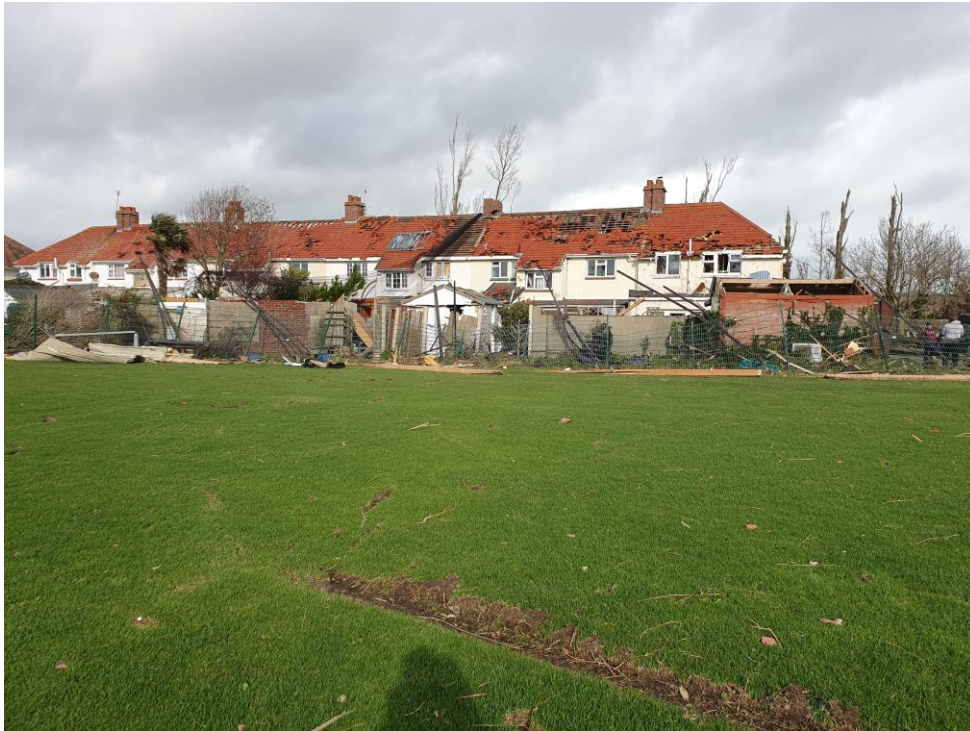
Figure 17: Houses on the northern boundary of Florence Boot Playing Fields where the internal bedroom wall blew down. The boundary fence can be seen to be badly damaged.
