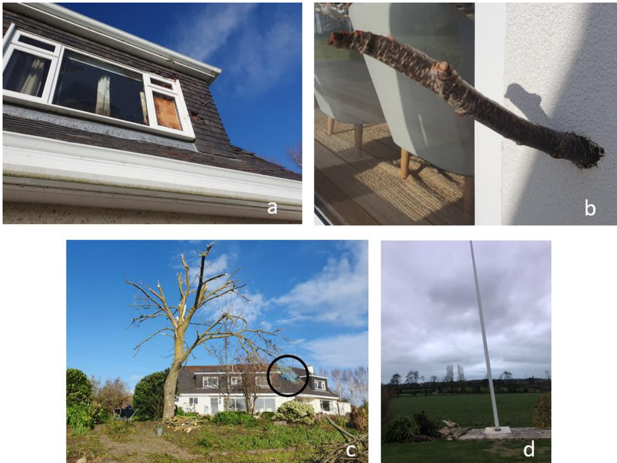
Figure 25: A property in Boulivot. a) Smashed window and embedded debris. b) Twig with estimated diameter 1cm embedded in render. c) View of house showing roof damage. d) Bent Flagpole which had partially been separated from its baseplate, separating partially from the baseplate. (credit Lee Battrick)
