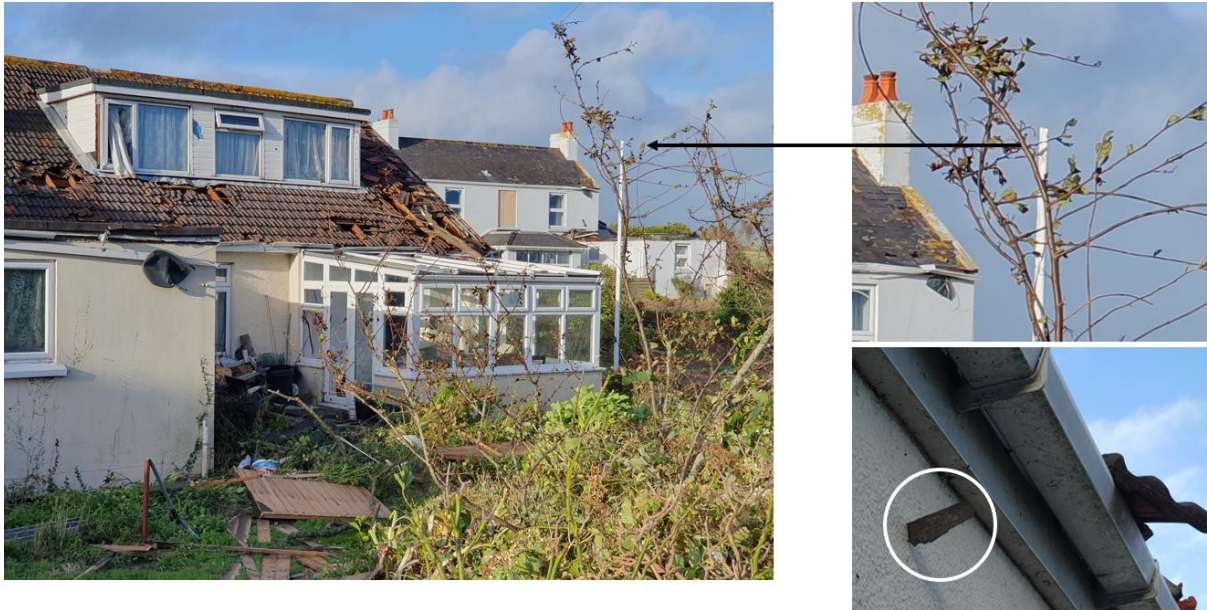
Figure 28: Property with embedded branch and a damaged flagpole and an example of embedded roof tile at another property along the La Route de la Hougue Bie.
