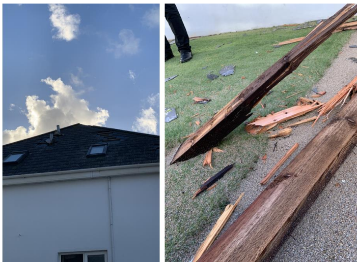
Figure 9: Damaged roof (left) and embedded roof timber in artificial lawn (right). Credit Angela Little.
