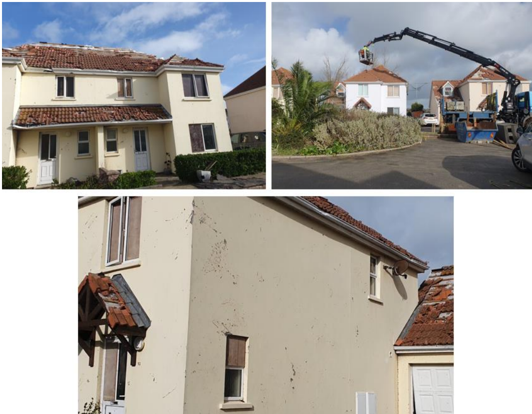
Figure 11: Typical damage to many homes in Florence Boot Cottages. Roof damage and deep gouges to the render.
