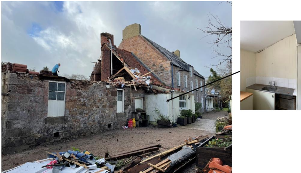
Figure 30: North face of the farmhouse (a) and attached barn (b). The farmhouse suffered tile damage, partially collapsed chimneys and blown out windows. The cream building is the lean-to extension, less well constructed building which appears to have shifted position. Credit Ian Tillotson.
