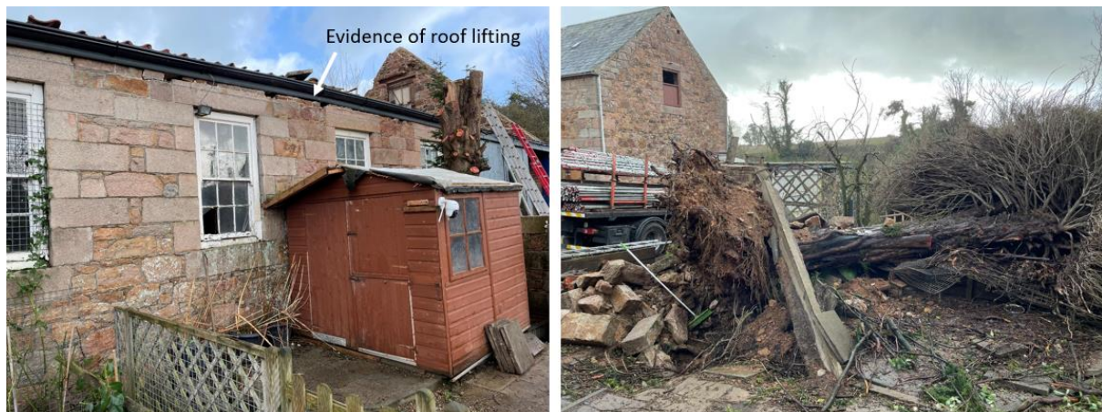
Figure 31: Evidence of the roof having lifted on the southern face of the farmhouse. A tree toppled towards the west.
