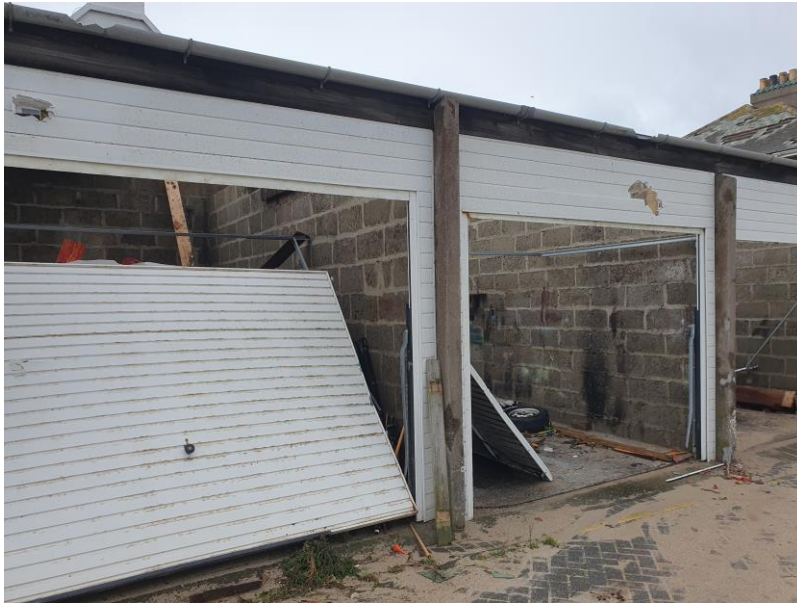
Figure 12: Block of garages with missing roof.
