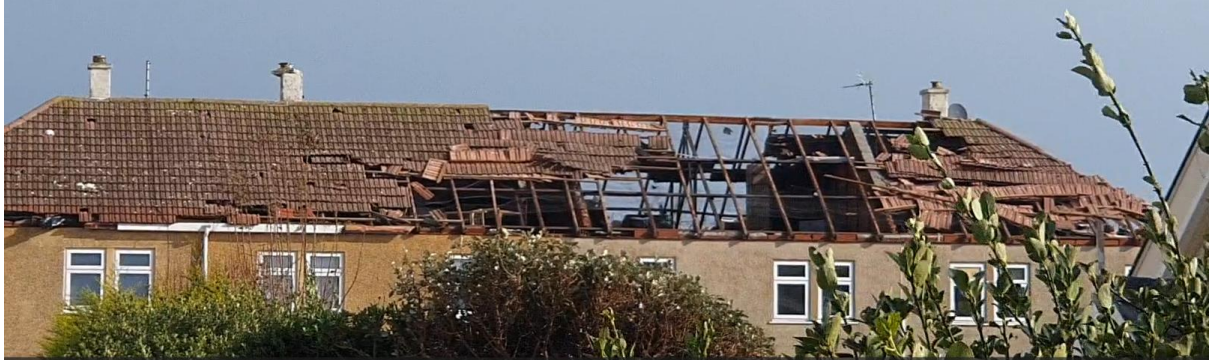
Figure 10: Homes behind St Nicholas with exposed roof joists.
