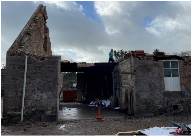
Figure 32: Attached barn (Figure 35 'b') showing roof loss and damage to remaining walls. View of the eastern end of the northern side. Credit Ian Tillotson.
