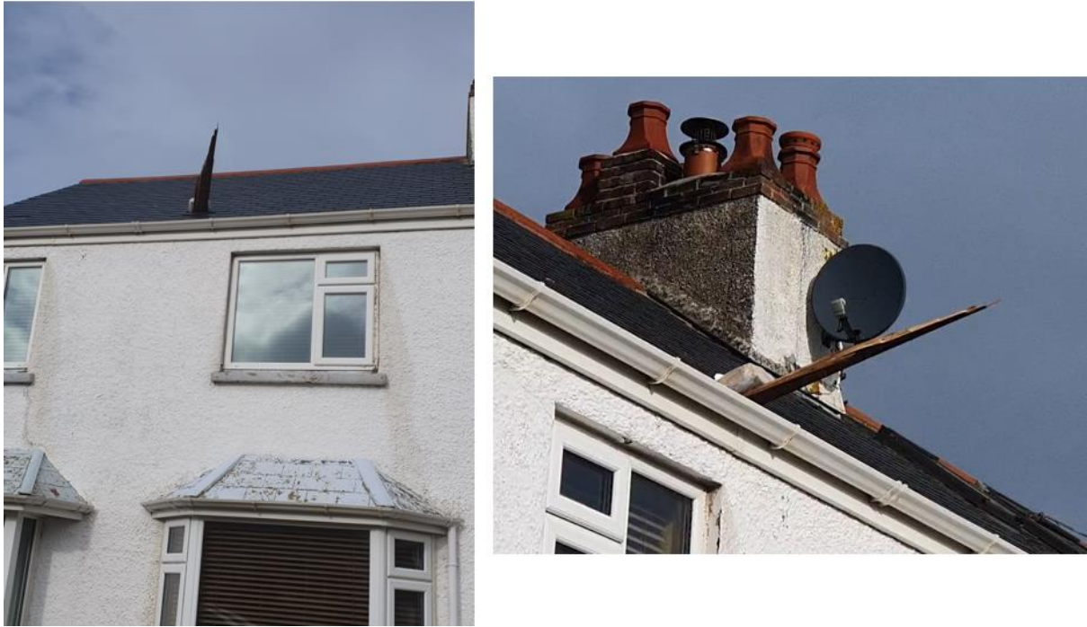
Figure 8: Two views of a property close to the sea front which appeared intact other than debris projecting from the south-eastern side of the roof.
