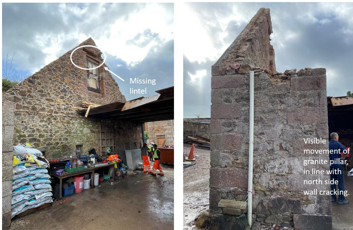
Figure 33: Closer detail of damage to the attached barn.
