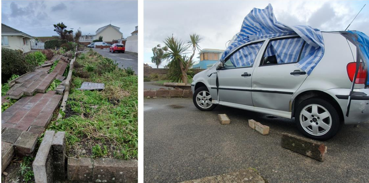
Figure 5: Collapsed garden wall and a damaged car parked by it.
