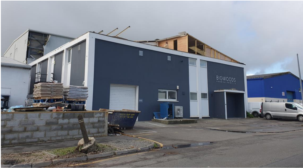
Figure 22: Partial roof loss from another warehouse in Rue Des Trading Estate.
