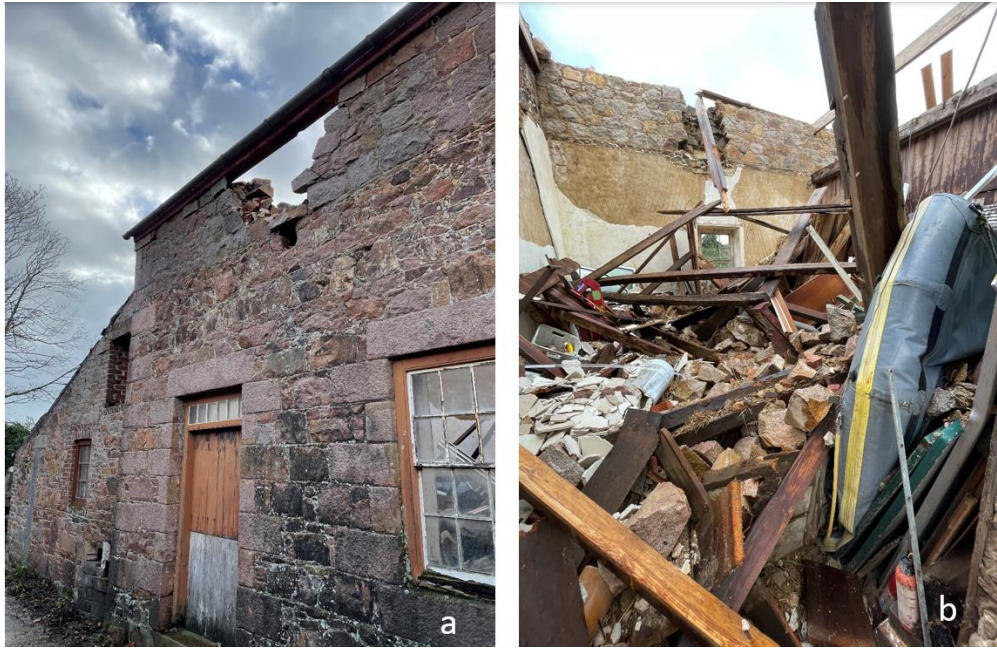
Figure 34: a) Damage to the north wall of the southern barn (Figure 29 'c') b) Inside the southern barn, showing the loss of roof and collapse of the gable end. Credit Ian Tillotson
