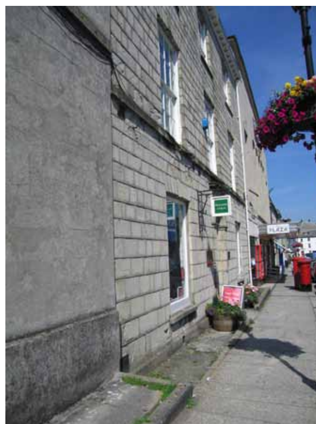
The removal of boundary treatment such as railings and walls can have a detrimental effect on the streetscape.
