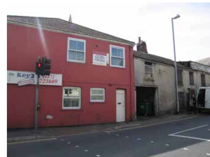
These buildings are in urgent need of repair: 14-16 St Clement Street
